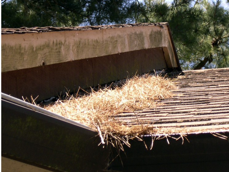
Figure 5. Vegetative debris accumulated at this roof-to-wall intersection. Ignition of this debris would expose the adjacent siding to flames, as well as the underlying sheathing above this stand-alone Class A roof covering. Depending on the overall roof design, the Class A roof covering could give the homeowner a false sense of security. Photo: Stephen L. Quarles.
