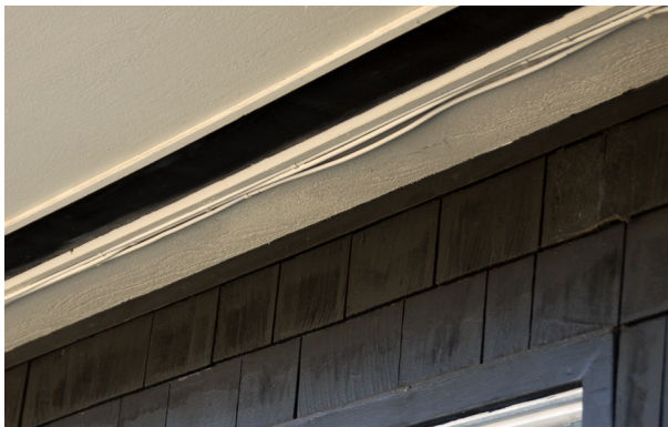
Figure 14. An example of a soffited eave, also sometimes called a boxed-in eave. Depending on the vulnerability of the vent, embers could enter into the soffit area. Vertical flame spread up the wall would make flame entry through the vent and into the attic more likely. Moving the vent away from the wall (closer to the edge of the roof) would make flame and ember entry less likely. Photo: Stephen L. Quarles.
