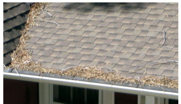
Figure 8. Debris accumulation behind a gutter cover device. The gutter is clear of debris, but the roof still should be cleared of debris. Photo: Stephen L. Quarles.
