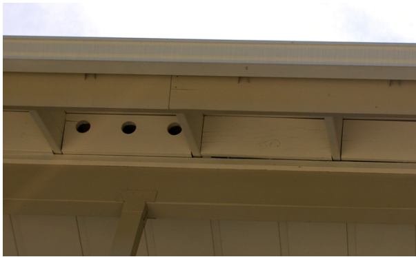
Figure 13. An example of open-eave construction. The roof rafter tails are exposed. The circular frieze-block vents shown here are typically located in the blocking. Note the gaps between the blocking and adjacent framing which would allow ember entry. These gaps could be caulked. Backer rod may be needed for wider gaps. The caulked joints should be inspected annually and failed joints repaired. Photo: Stephen L. Quarles.
