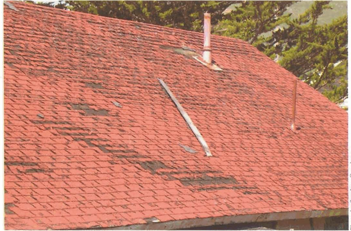
Photo by Stephen Quarles Worn out shingles lose their effectiveness as both fire and moisture resistant materials. Roof coverings must be replaced once they have reached the end of their useful service life.
