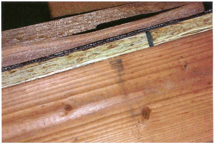
A fire retardant treated wood shake roof with Type 72 roll roofing as a fire barrier material located between the wood shakes and the oriented strandboard sheathing.
