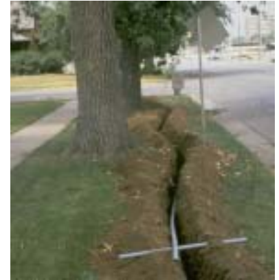
Figure 6: Trenching near trees can severely damage root systems.
