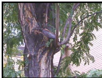
Figure 10. This adventitious sucker growth from a reduction cut is structurally unsound and prone to storm damage as it grows.
