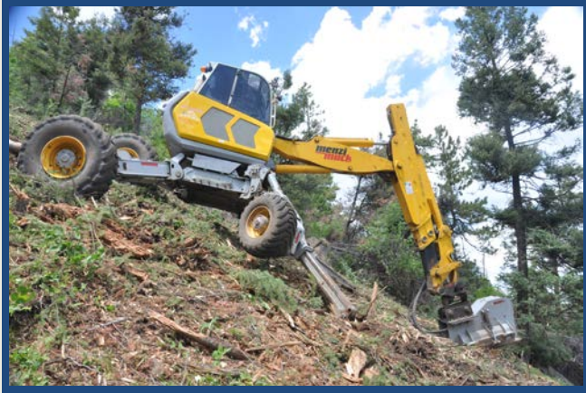
An all-terrain excavator removes fuels from a steep slope of the Rampart Range, Douglas County.
